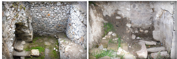
Fig. 10 Fountain deteriorations (material losses, vegetation on the sides, dampness, mossiness problems from the ground etc.)
