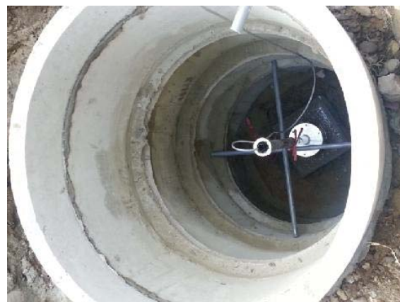
Fig. 2 A seismometer was mounted on the concrete foundation with a depth of 2 meters in the second stage
