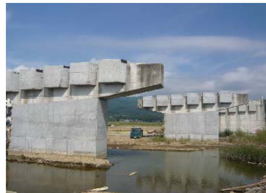
Fig. 5 Damaged Numata-Kosen bridge during Tohoku Tsunami
