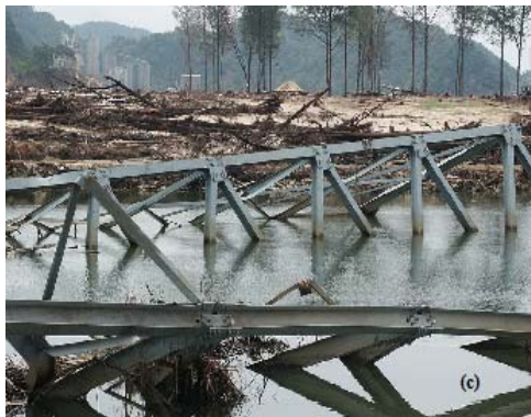
Fig. 2 Bridge damage due to tsunami attack in Banda Aceh (a) Total Wash-Away of Deck [7] (b) Excessive Deck Displacement [12] (c) Damaged steel truss bridge with damaged cement plant in the background in Lhok Nga, Banda Aceh
