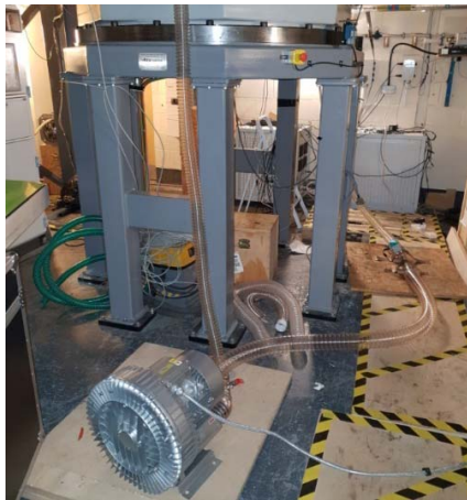
Fig. 6 SC-7500 fan connected to floor side circulation system
