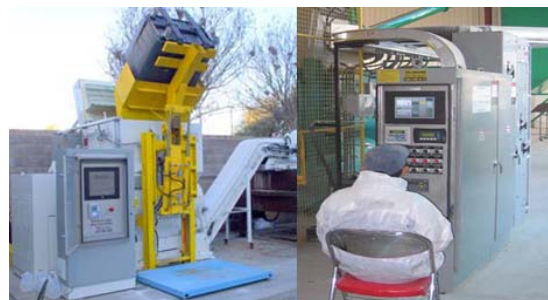
Fig. 1 PIWS non-burn HCRW Treatment System [7]
