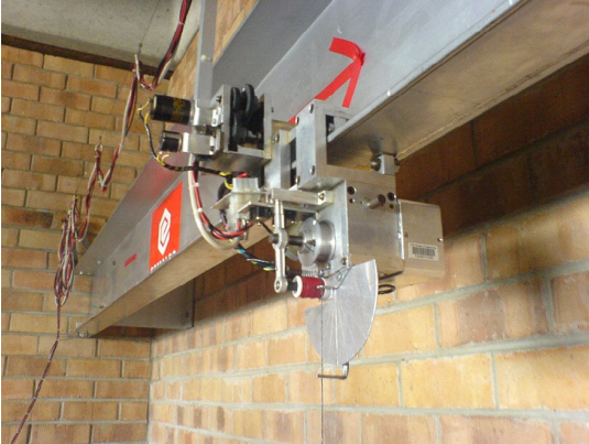
Fig. 1 Gantry crane system
