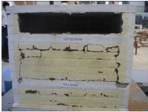
Fig. 14 Final Collapse – Model S2
