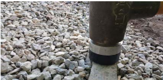
Fig. 7 The hammer impact
