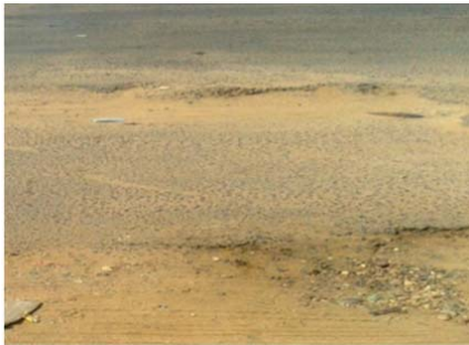
Fig. 3 Severe potholes and damaged edge in Shambat west road
