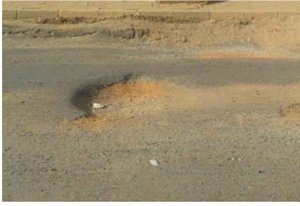
Fig. 2 Severe rutting leading to large potholes in Algaba road
