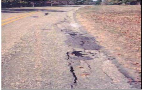
Fig. 1 Longitudinal cracking and failure, [19]
