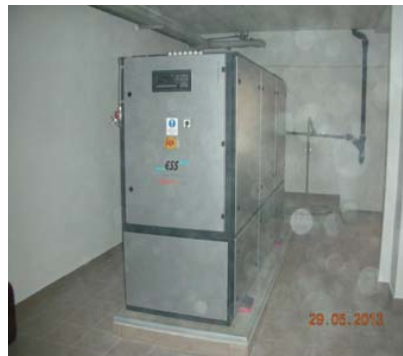
Fig. 5 Cogeneration unit 55kW
