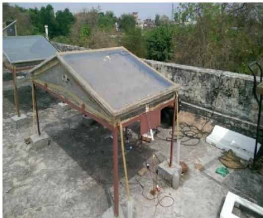
Fig. 1 Experimental Setup of MDSBMSS installed at MNNIT Allahabad
