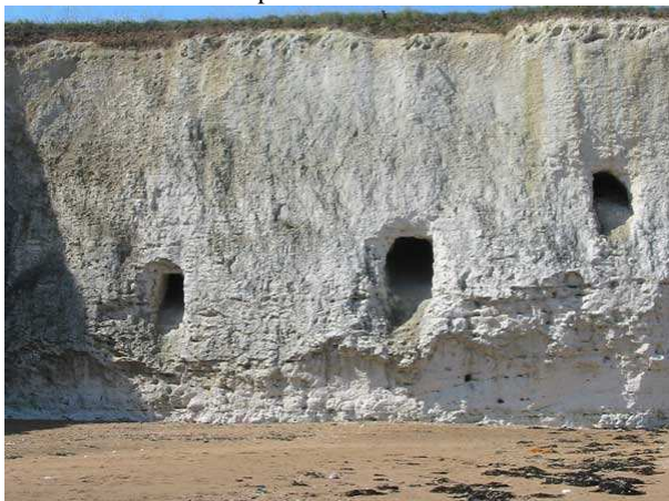
Fig. 3 Cavities of typical piping / sapping erosion [6]
