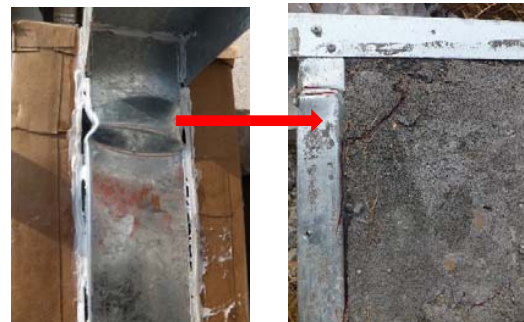
(c) Local buckling of W-3 CFS
