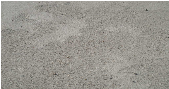
Fig. 5 (a) Spalling of pavement
