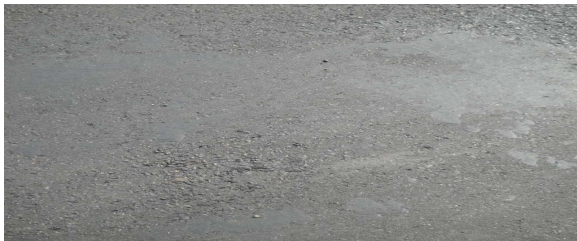
Fig. 5 (b) ) Bleeding of asphalt
