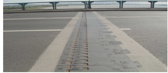
Fig. 4 (a) Joint fill with dust
