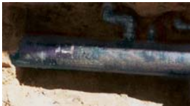
Fig. 3 Surface oxidation of ductile iron pipe buried in a corrosive soil.
