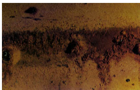
Fig. 2 Ductile iron pipe corrosion
