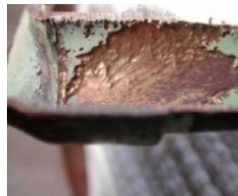
Fig. 10 Copper pipe corrosion
