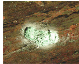
Fig. 8 Pitting corrosion of copper pipes
