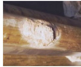
Fig. 6 Galvanic ringworm corrosion
