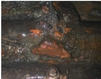
Fig. 14 Culvert pipe corrosion
