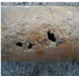
Fig. 5 Corrosion on a ductile iron distribution water main
