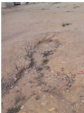
Fig. 3 Erosion in the area
