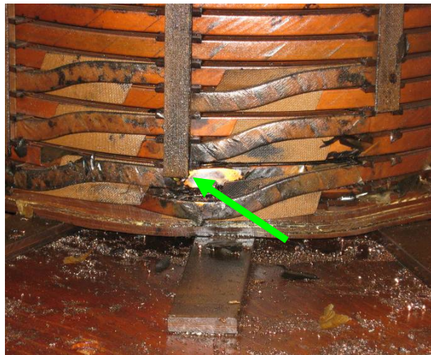
Fig. 12: Arrow shows the arcing spot
