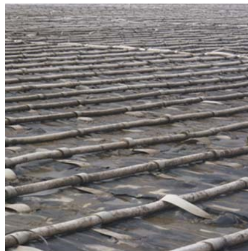
Fig. 4 Plastic pipes laid horizontally for water discharge and to support the membranes
