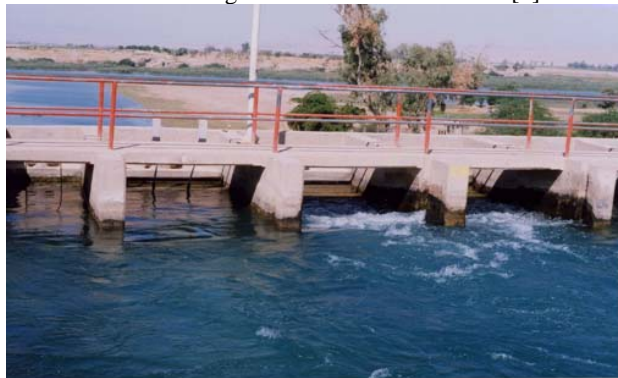
Fig. 2 The pumping station which feeds the Sabilli command area
