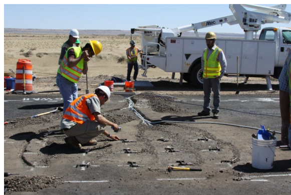
Fig. 3 Installation of horizontal strain gauges
