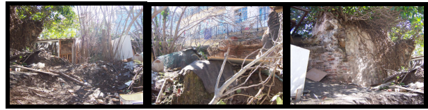
Fig. 11 The bath's interior filled with soil and garbage, the upper parts of the bath walls completed with random stones and the trees blooming out of these - 2014
