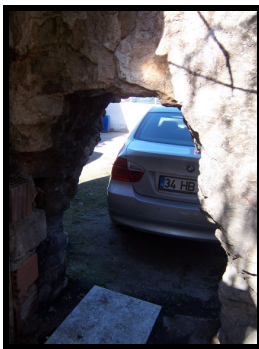
Fig. 10 The gap opened on the body wall of the bath by the enterprise - 2014
