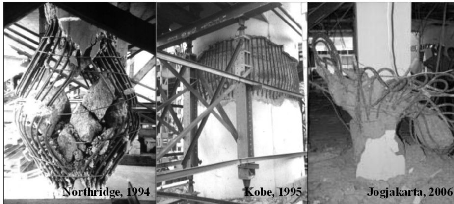
Fig. 1 The failure of structure in vertical earthquake
