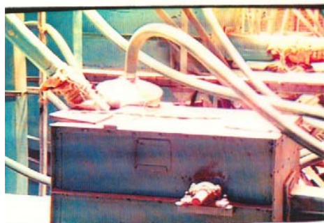
SUCTION FROM WOODEN FRAME CONTAINING SHELLER FAN
