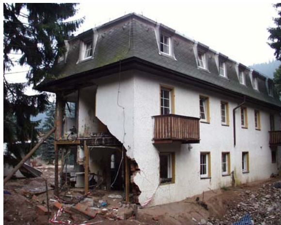
Fig. 1. Example of a close to collapse building with intact floor parts. Photo: Michael Markus.
