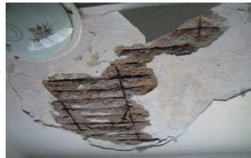
Fig. 3 Spalling of concrete
