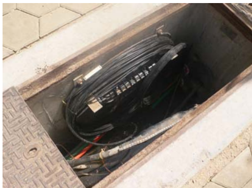
Fig. 4 Mounted splice closure at one of the outside plant intersections
