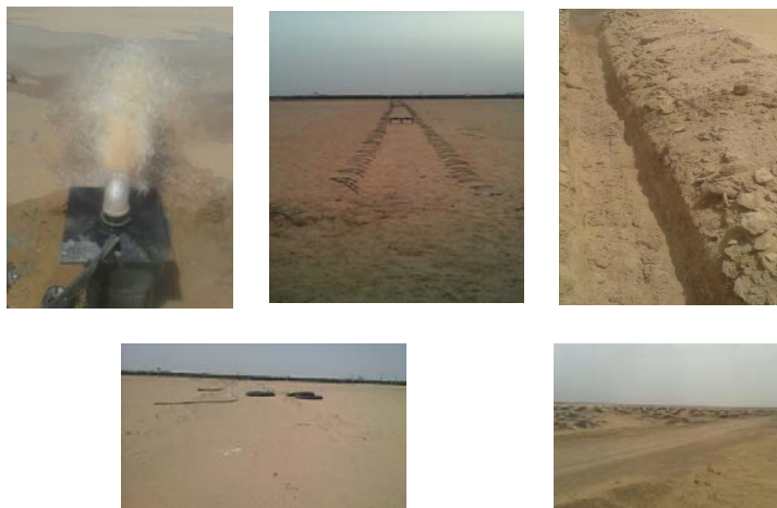
Fig. 9 (c) Various pictures of the land being prepared and ready for use as a field test environment
