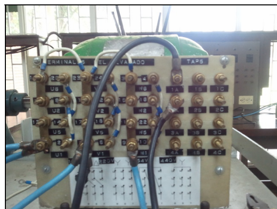
Fig. 5 Connection board of the motor under test
