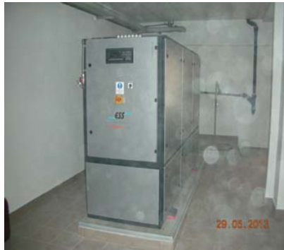
Fig. 5 Cogeneration unit 55kW
