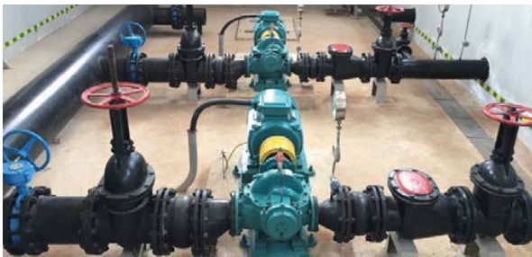
Fig. 1 Circulating Water Pump
