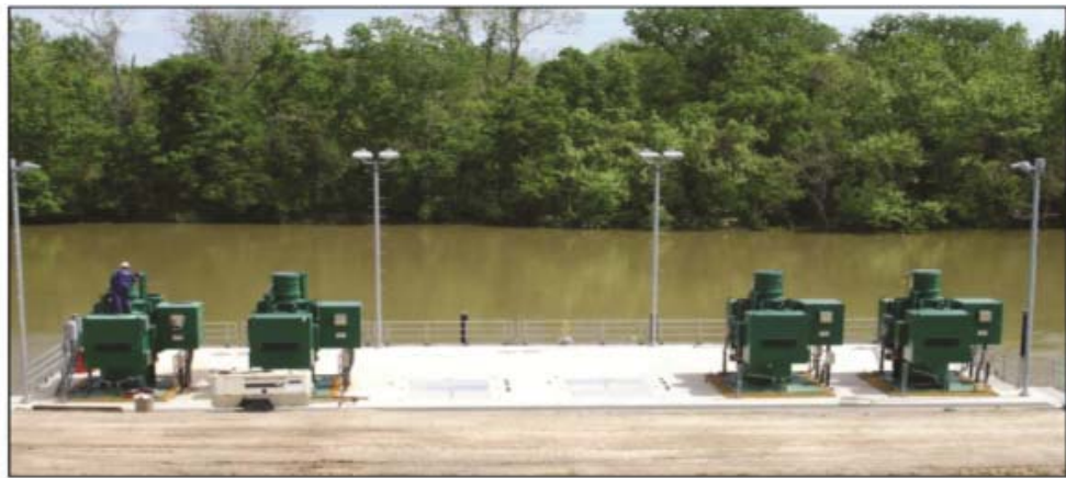
Fig. 6 Site location's existing Pump station
