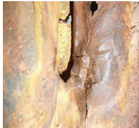
Fig. 1 Cracks at fin tip of tubes membrane
