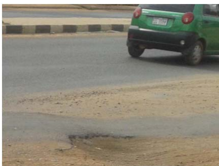
Fig. 4 Severe surface damage along the edge lane in Alarbeen road
