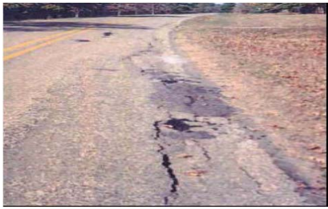
Fig. 1 Longitudinal cracking and failure, [19]
