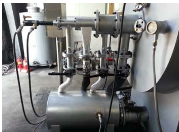
Fig. 4 Picture of the Pet-coke burner
