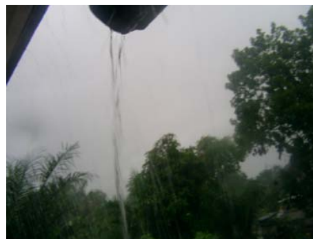
Fig. 3 Water falling from the roof gutter
