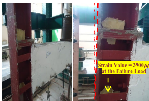
Fig. 14 SP3; Beam flexural cracks and column deformed shape
