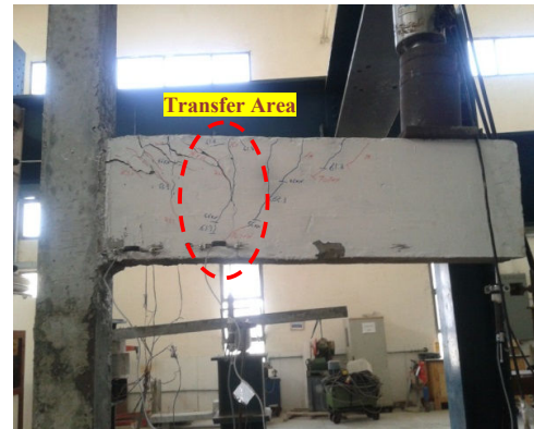
Fig. 15 Cracks at the failure of SP4
