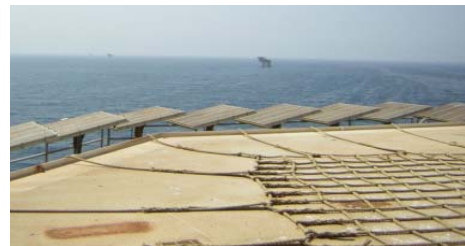
Fig. 2 Solar panel on unmanned platform
