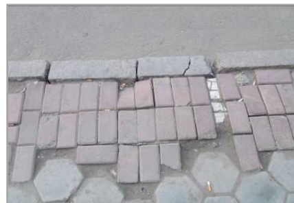
Fig. 16 (a) Damaged pavement on the Ceramic Street logos on the Ladies' Street
