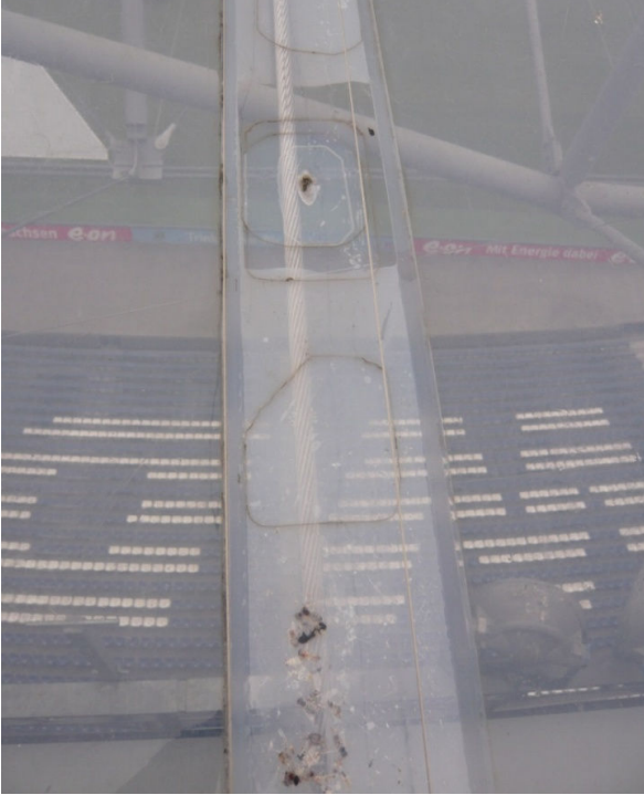
Fig. 17 Picture of Hanover stadium roof – patches on a cable pocket and insects
