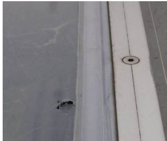
Fig. 16 Picture of Hanover stadium roof – holes close to an edge
