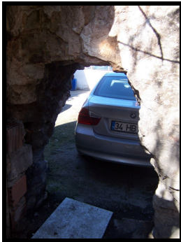
Fig. 10 The gap opened on the body wall of the bath by the enterprise - 2014
