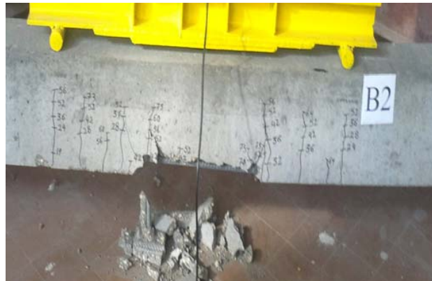
Fig. 5 Typical splitting failure for beam specimens without confining transverse reinforcement
