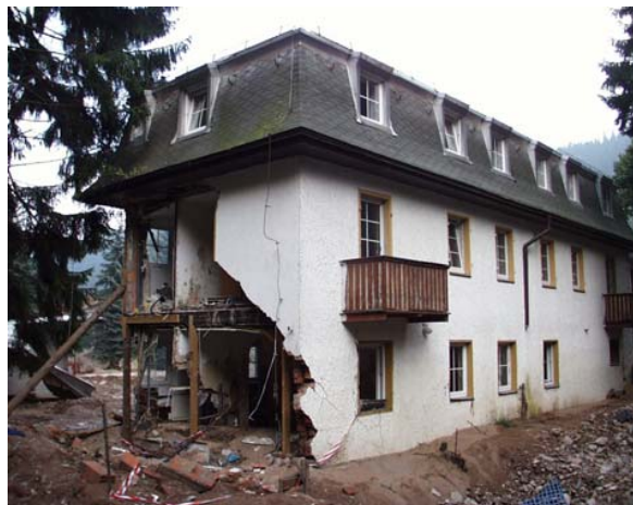
Fig. 1. Example of a close to collapse building with intact floor parts. Photo: Michael Markus.
