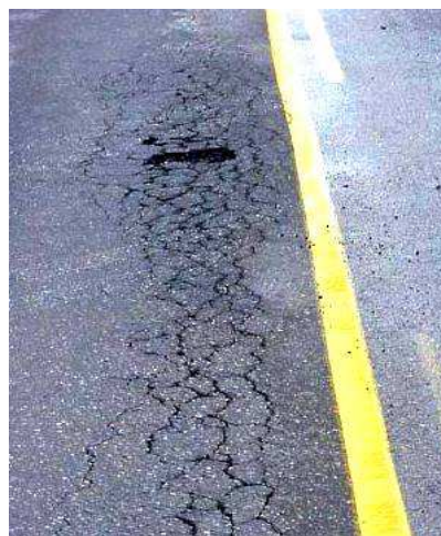
Fig. 4 fatigue causes pothole
