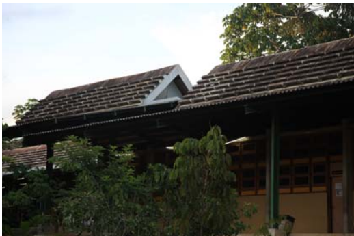
Fig 9. Campus UFAM, Manaus. Concrete roofing, with openings to allow air flow and improved thermal pefromance, while protecting from intense solar radiation and rains.
