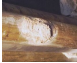
Fig. 6 Galvanic ringworm corrosion
