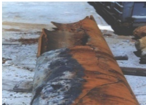
Fig. 1 Ductile iron pipe failure
