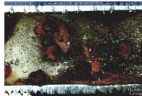
Fig. 7 Corrosion of galvanized potable water piping
