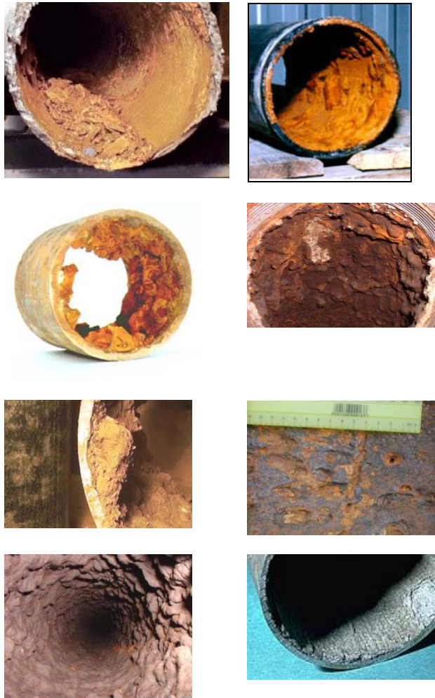
Fig. 17 Different cases of internal corrosion in metallic water pipes
