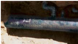
Fig. 3 Surface oxidation of ductile iron pipe buried in a corrosive soil.
