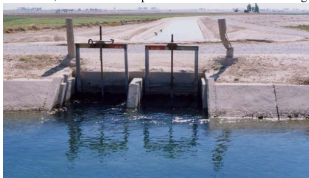
Fig. 3 A cross-regulator in a main canal
