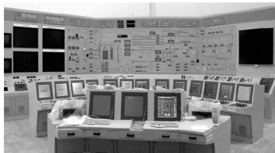
Fig. 1 Modern Main Control Room of the NPPs
