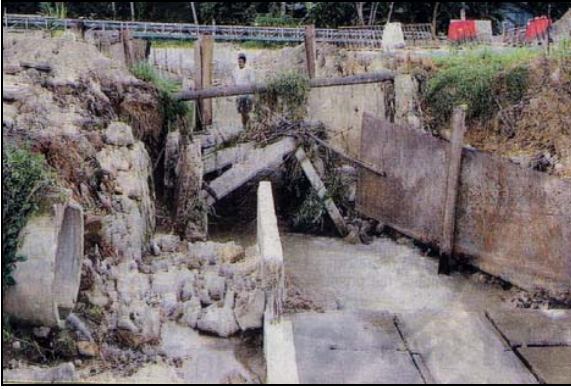
Fig. 6 Bridge in Seremban, Negeri Sembilan collapsed due to heavy rain and flooding [20]
