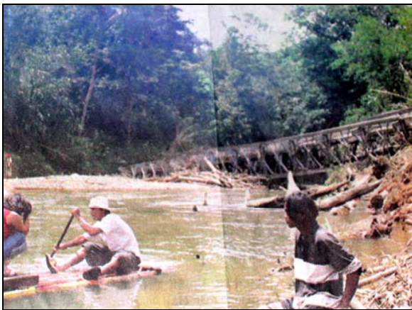
Fig. 8 Bailey bridge collapse due to heavy floods [20]
