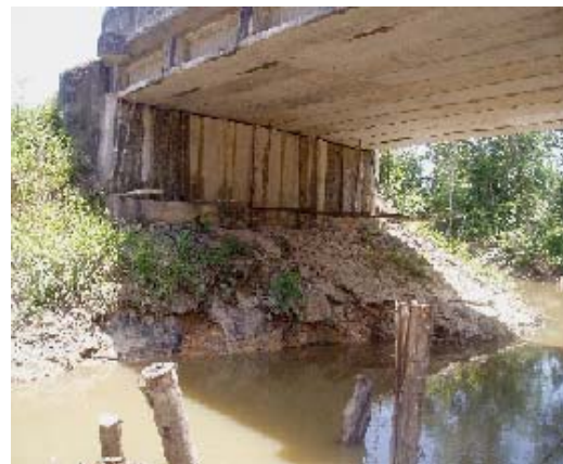
Fig. 5 Bridge failure due to scouring at Bokah Rasau Stungkor Road, Kuching, Sarawak [20]
