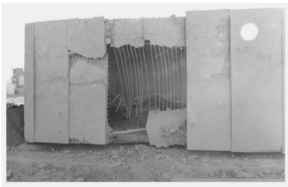
Fig. 3 Breaching Failure of the Beam in the form of Bursting [5]
