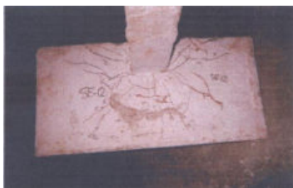
Fig. 2 Crack pattern as exhibited by Se-12
